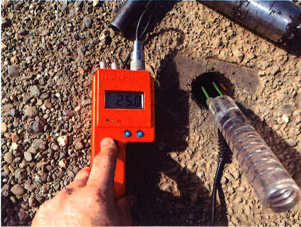
Moisture testing at Test Core # 2 indicated that the insulation contains moderate levels of moisture.
