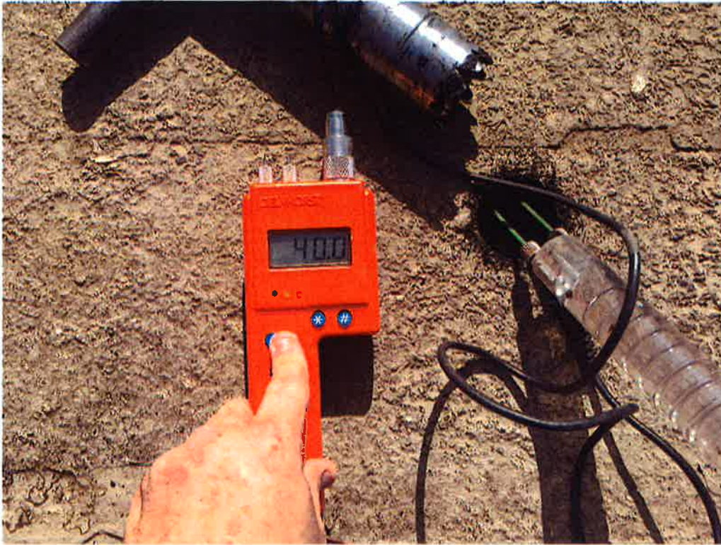
Moisture testing at Test Core #1 indicated that the insulation is saturated. Standing Water was observed in the bottom of the core hole. A reading of 40.0 is the highest possible reading provided by the instrument in terms of moisture content.
