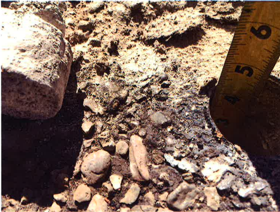
View of Test Core # 3 The moisture reading for the insulation was 40, indicating the insulation was saturated with moisture
